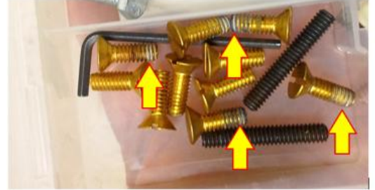
Galvanic Corrosion on Brass Cover Plate Screws
